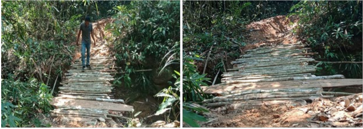
Making a wooden forest bridge over a seasonal river in the Cardamom Rainforest Landscape; part of 155-km of forest trails improved during this reporting period,
